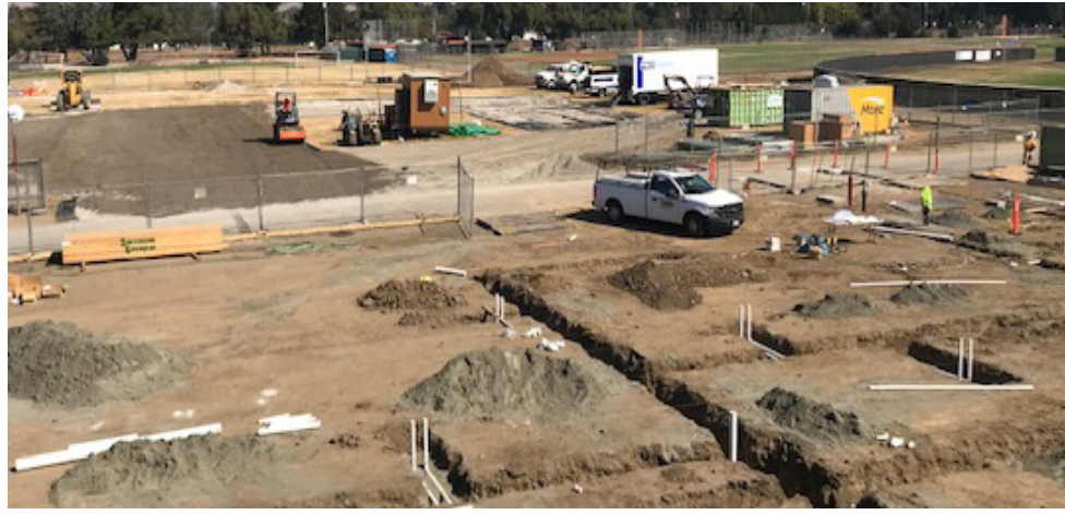
Workers outside of Washington's E-Building continue construction on the new science wing of campus. This project demonstrates the school's effort to accommodate the influx of students enrolling at Washington.
